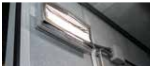
Internal lighting system
